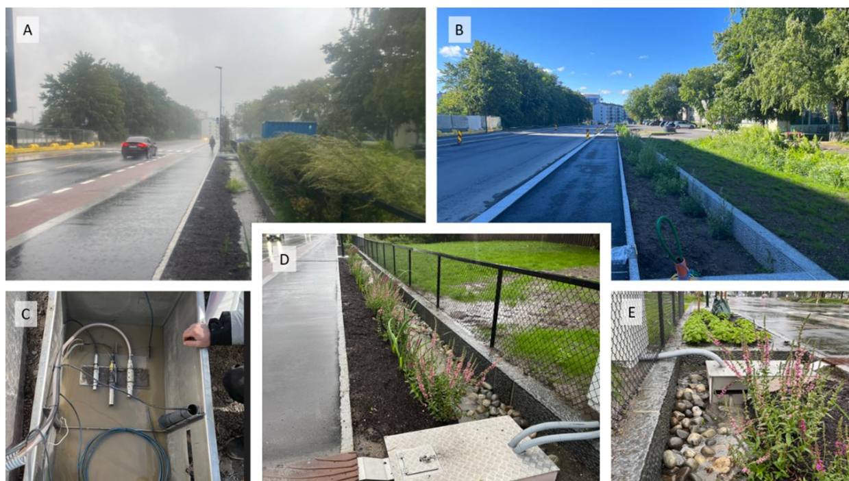
Figure 7.1 A) The road and the raingarden during a heavy rain event (August 2023), B) the raingarden under construction (summer 2022), C) sensors installed in the influent monitoring box, D) the raingarden and the influent monitoring box, E) the raingarden and the influent monitoring box showing water flowing over the v-notch.
