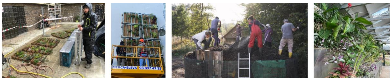
Figure 4. Installation of the GRETA ® green wall for greywater treatment and reuse in St. Quirze, Barcelona, Spain - Social Housing, one of the pilots of the MULTISOURCE project (images 1 and 2 from the left, photo credits: ICRA)
